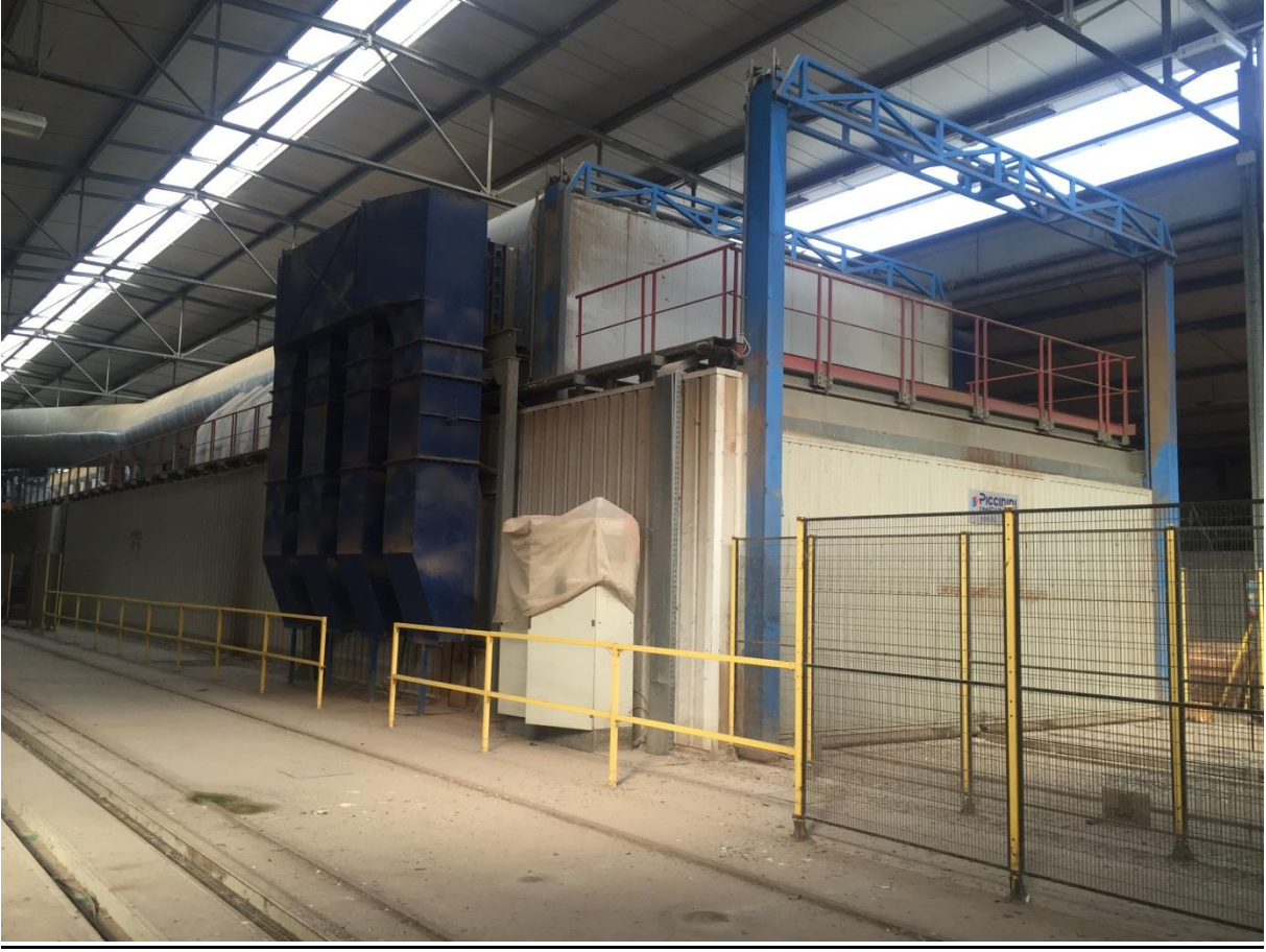
KILN (PICCININI IMPIANTI, ITALY):
